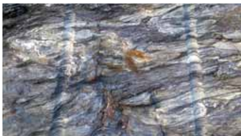
As a consequence of the motorway construction, the escarpments show their shale composition
