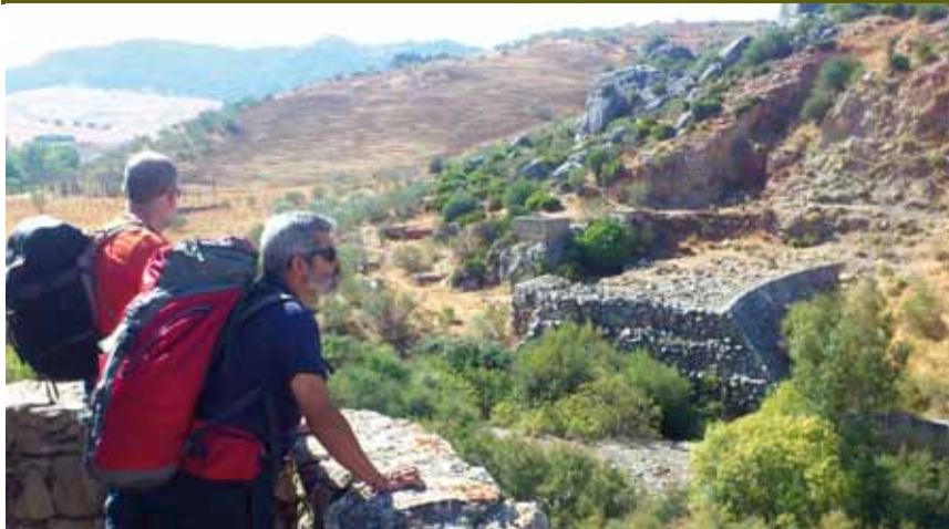
The retaining wall of the unfinished dam of Río Turón, in La Laja
