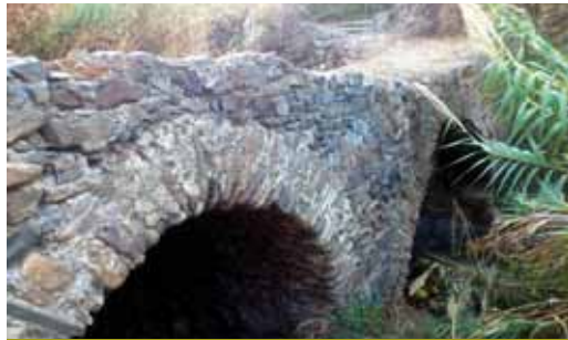
Puente de las Animas with its two arches of stone blocks and mortar
