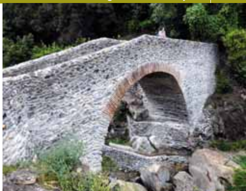
The Puente de Salares, which gives access to the village, has been restored to its former splendour
